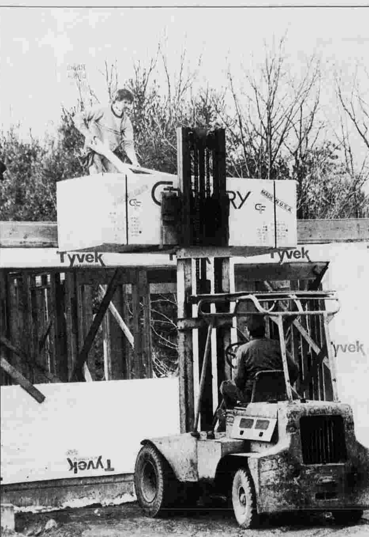
GOING UP — Ken Beaulieu, driving the forklift, raises a load of plywood to Scott Hitchcock who works on the roof. Beaulieu is from Manchester. Hitchcock lives in Andover. The warmer weather this week has been a boon to contractors.
