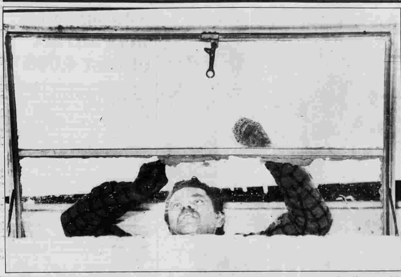
FRAMEWORK — Mike Margolyou of the Rockville section of Vermont puts the finishing touches on a window he replaced at the Connecticut Bank and Trust Co. office on Main Street in Windsor. He works for A-1 Glass Co. of South Windsor.
